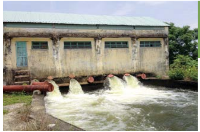
Figure 1.41: Tu Cau pumping station, Vietnam. (Tran Thi Ha Van)
