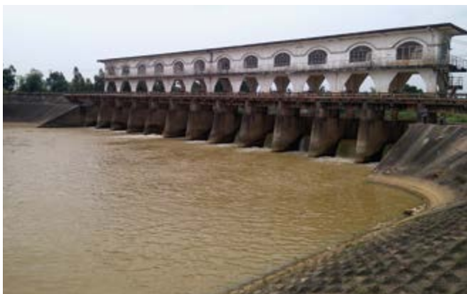
Figure 2.7: An Trach barrage on the Vu Gia river, Vietnam. A similar weir could be constructed further downstream as permanent protection against salt water intrusion (measure No. 3). (Trinh Quoc Viet)
